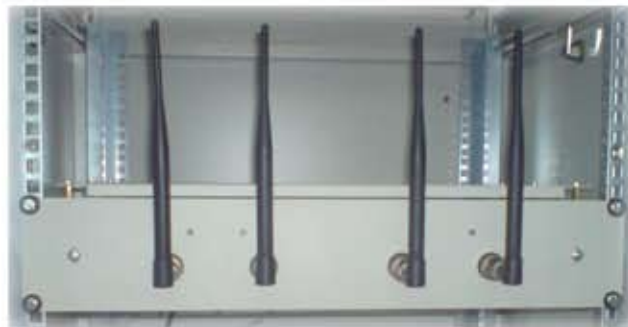
Low Power Rack Installation
